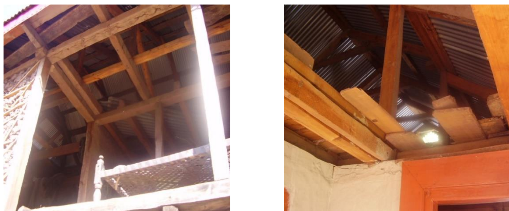
Figure 9: Practice of tower roof in an under-construction house in Kaimanja, Muzaffarabad. Source: Author
