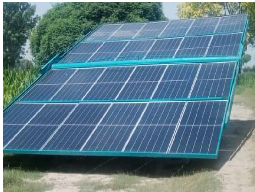
Fig 3: Solar Panel plates for solar tube well.
