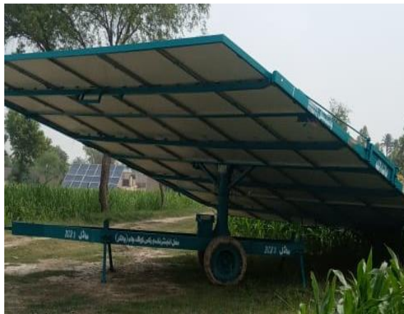
(A) Operating Condition Stand
