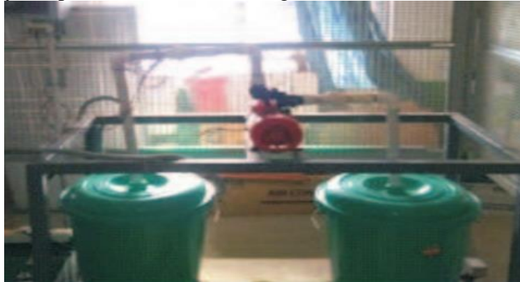
Figure 7. Solar powered AC water pumping system
