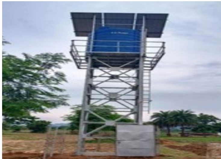
Figure 6. Ground mounted solar PV irrigation system
