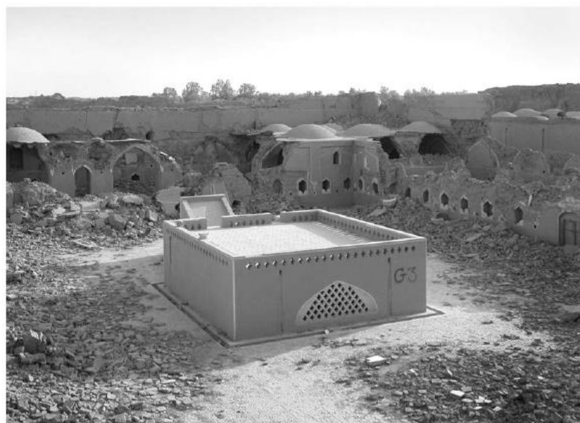
Fig. 18: An example of damage to the buildings of the Bam Citadel complex before (above) and after (below) the 2003 Bam earthquake (Langenbach, 2005)
