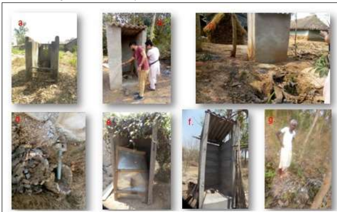
Figure 9 : a. The roof of toilet has broken in one year after construction. b. & c. Plaster is opening from the newly constructed toilet wall in Lailamdi village (Bundwan block). The pit on the toilet is open at the back, as a result filling in other garbage. d. In the village of Tasgram (Bundwan block), the structure of a family's toilet pit is being torn down. e. The door of toilet slammed in the air. The
