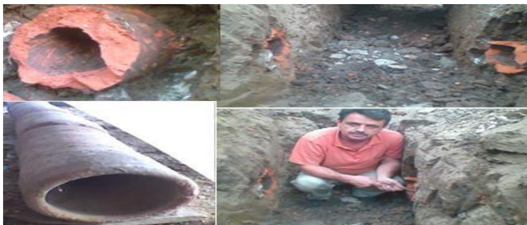
Figure 6. View of ceramic water \pi pes in the canal in a narrow and wide profile at a depth of 55 cm-Bostanisht., 1980 and 2010 (N. Kamberi-Zhunica), III century A.K (After Christ).
